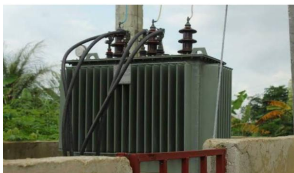
Plate 4: Electricity Facility in Okekoto Community, Agege LGA (Transformer).
